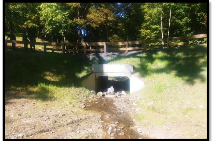
Scenic Hudson Land Trust received a grant to improve the aquatic organism passability and reduce the flooding hazard of this vital piece of infrastructure.
