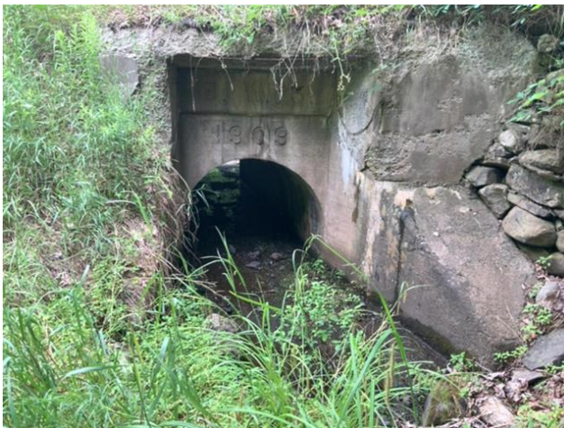
An example of a crossing that is aging on Atwood Road. Local ID: LEW_902
