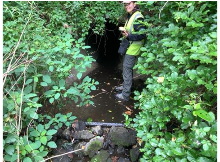
An example of a shallow crossing on Miron Lane. Local ID: LEW_011
