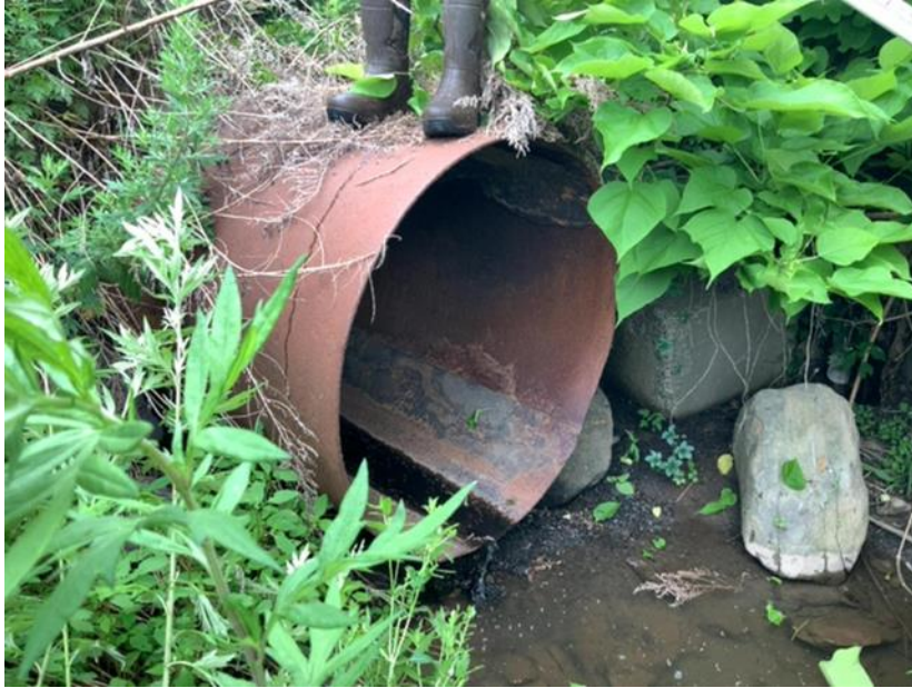
An example of a crossing that lacks natural substrate on Atwood Road. Local ID: LEW_030
