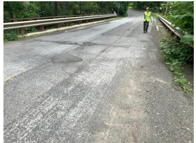
An example of road deterioration on Atwood Road. Local ID: LEW_029
