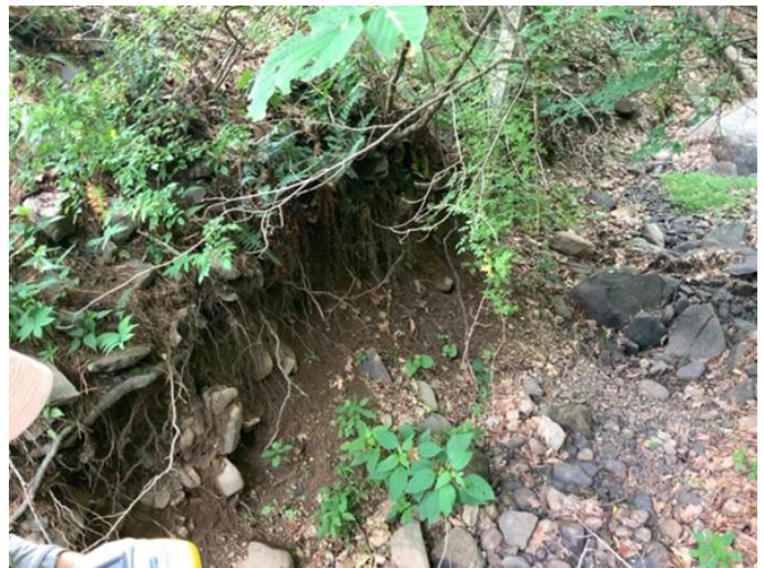
An example of erosion caused by a crossing on Atwood Road. Local ID: LEW_902
